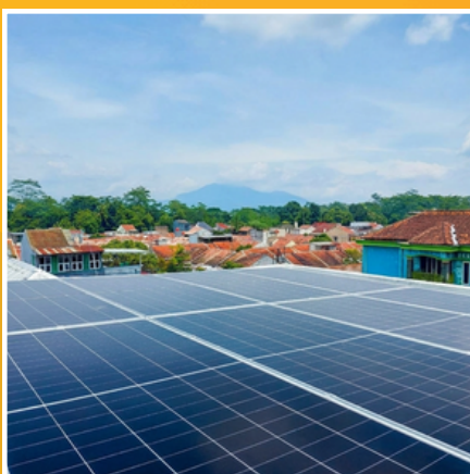
Salatiga - Jawa Tengah 8 Panel | 5 kWp
