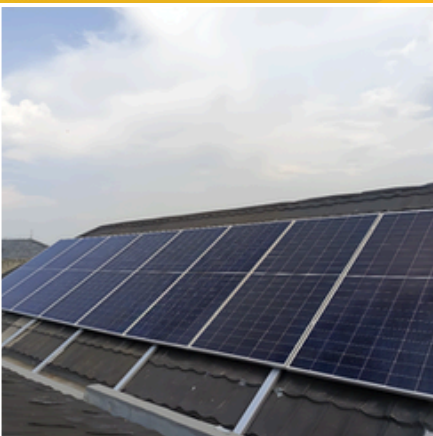
Serang - Banten 8 Panel | 5 kWp
