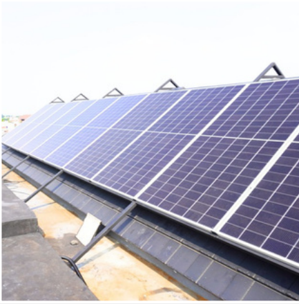
Matraman - Jakarta 42 Panel | 26 kWp
